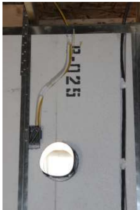
Figure 4: Electric wiring easily cut into foam panel
