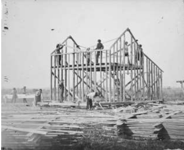
Figure 1: Ten men building a wood frame house on a Omaha Reservation in Nebraska in 1877
